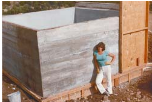
I just finished putting a coat of “Thoroseal” on the inside of the holding tank.
