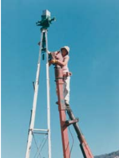
Boom truck stood the windmill up. I'm disconnecting the chain and hook 25 feet up.
